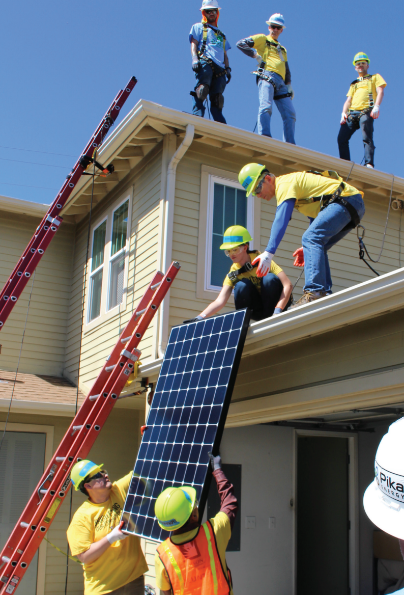
Photo courtesy of Grid Alternatives
